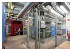
Power receiving equipment
